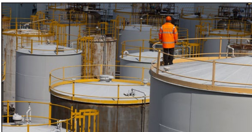
External pitting (corrosion) on carbon steel vessels is inevitable and can eat away the wall thickness if untreated. Anti-corrosive paints can be especially helpful in inhibiting external corrosion
